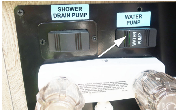
Water pump switch location on Water Center Panel behind rear doors. T36B -Typical View
