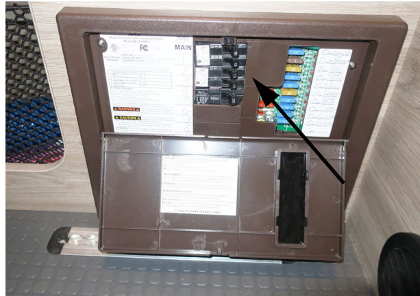
Ensure the breakers are in the “ON” position (flipped to the right hand side as shown above). -Typical View
