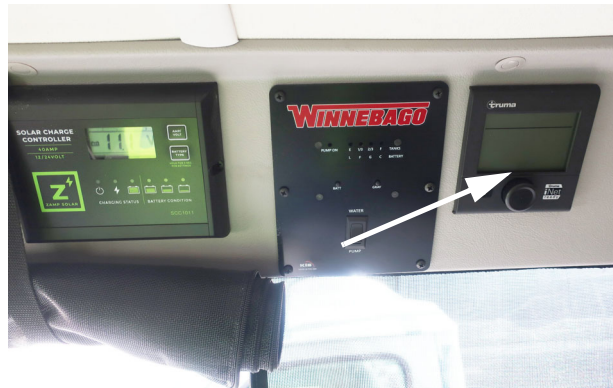
Water heater controls location on Systems Monitor Panel (T36A shown- T36B located in same position.) -Typical View
