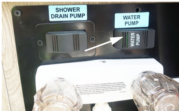
Pump switch T36B -Typical View
