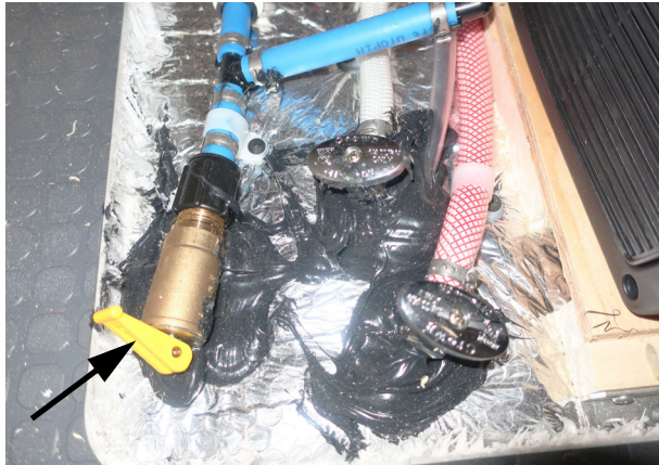
Water Heater drain valve (Located in the dinnette shown in the closed position). -Typical View
