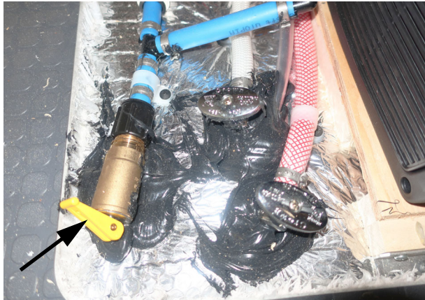
Water Heater drain valve (Located in the dinette shown in the closed position). -Typical View
