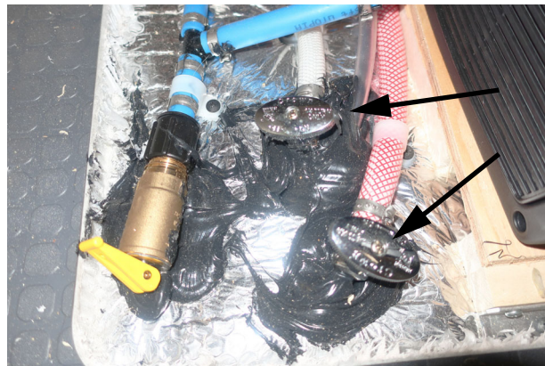
Fresh Water drain Valves T36B (Located in the dinette shown in the closed position). -Typical View
