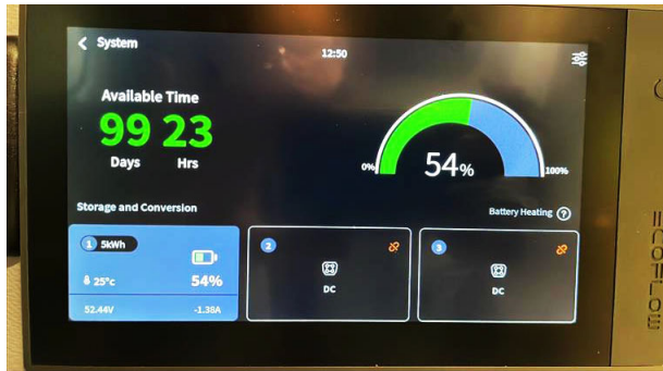
Selecting the System from the main menu will display available time, battery charging/discharging, battery state of charge (SoC) percentage, and temperature. -Typical View
