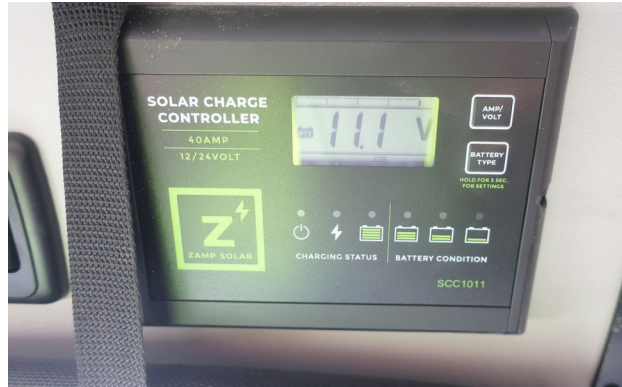
Solar Charge Controller (Located near the Systems Monitor Panel) -Typical View
