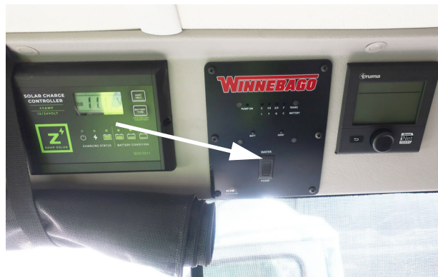
Water pump switch location on Systems Monitor Panel (T36A shown- T36B located in same position.) -Typical View
