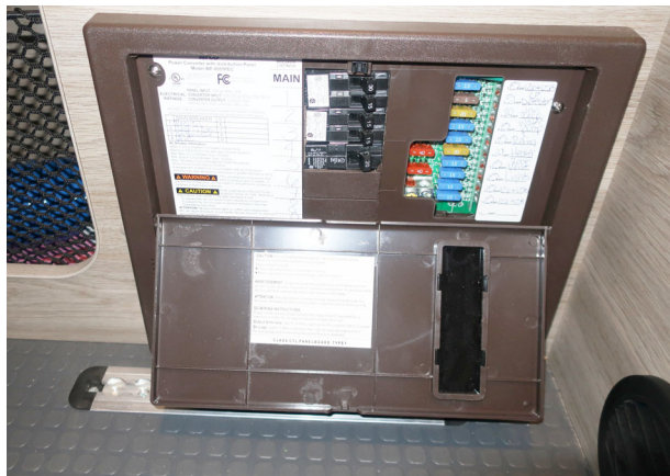
120-Volt Circuit Breakers -Typical View
