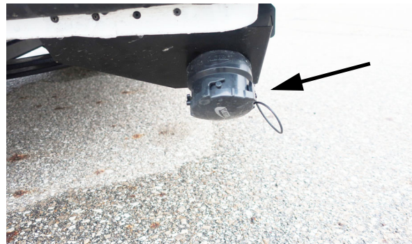
Sewage Drain Outlet
