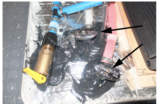
Fresh Water drain Valves T36B (Located in the dinette shown in the closed position). -Typical View
